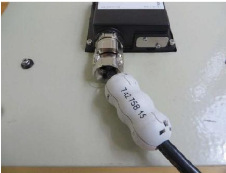
Figure 8: Ferrites on the PLC J-Box side
