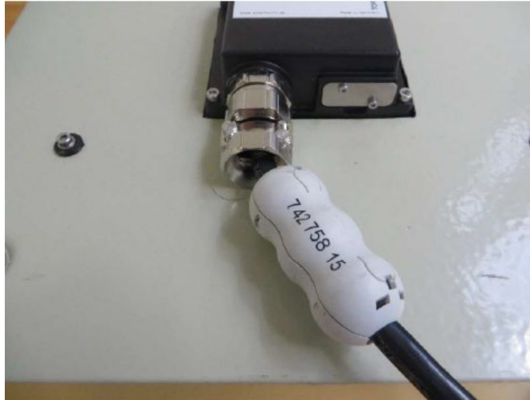
Figure 8: Ferrites on the PLC J-Box side
